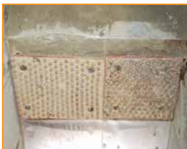
Discharge Chute Primary Crushing
